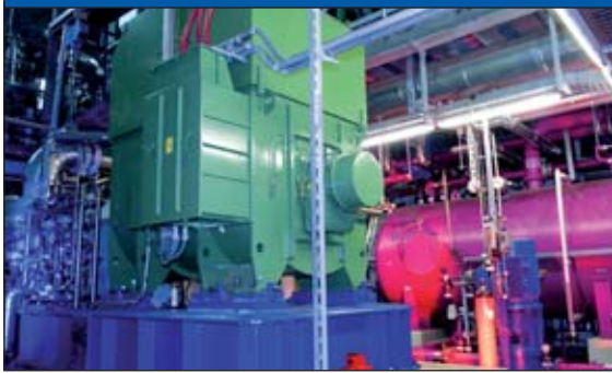
Fig. 9: Generator and ammonia tanks
